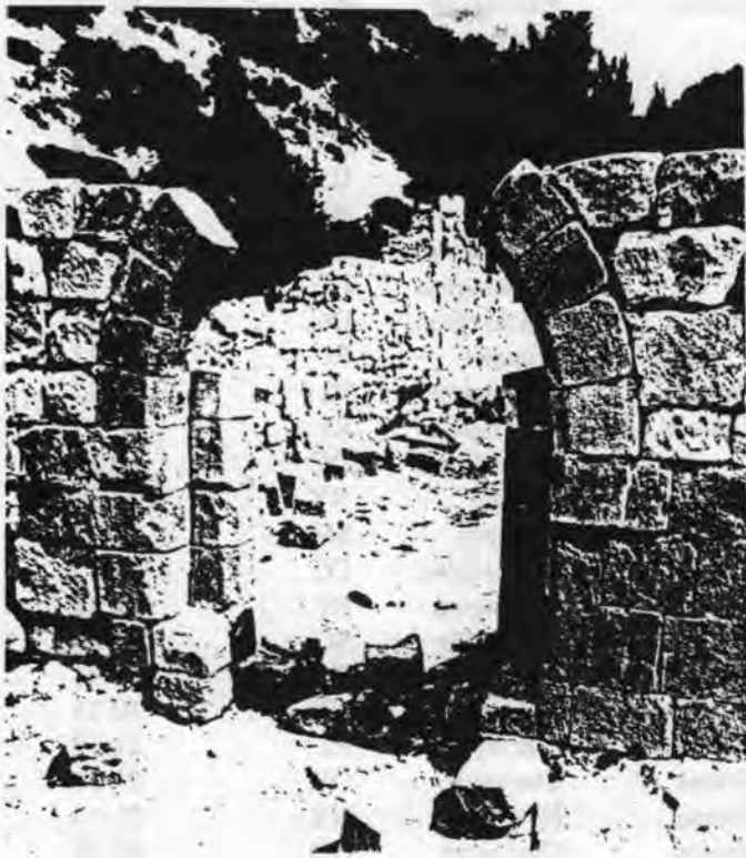
Chapel Entrance Arch After Vandalism
